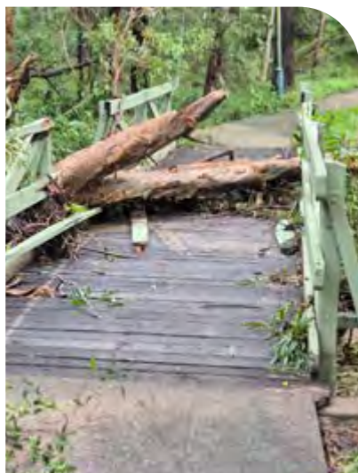
Cyclone damage in Cornubia Forest Park.
